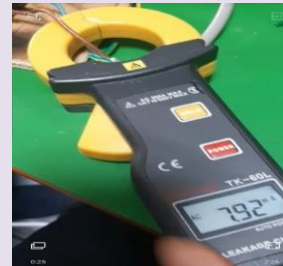
Before installing ENSPD ( 7.92mA)
