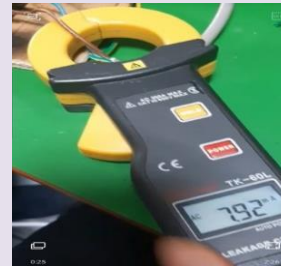
Before installing ECSPD ( 7.92mA)
