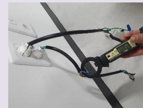
Before installing ECSPD ( 22.9mA)
